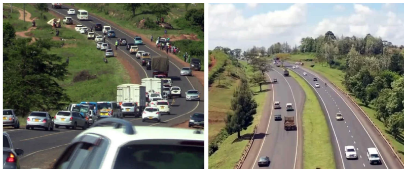
The Kenol-Sagana-Marua highway was a single-lane bitumen paved road. It is now being upgraded to a two-lane dual carriageway to ease traffic flow.
