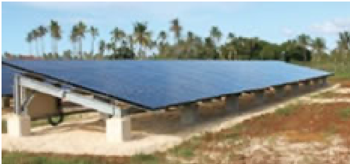
A solar power generation facility in Tonga
