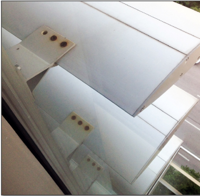
EXAMPLE OF FASTENER, CORROSION, AND FAILURE ON ARCHITECTURAL SUN SHADES. - IMAGE COURTESY OF USACE, OMAHA DISTRICT.
