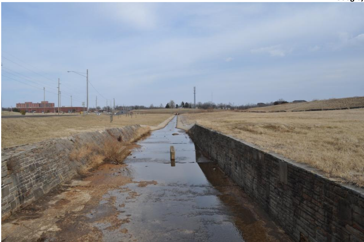
Photo 1. Current Stormwater Conveyance Method (Corner of Nebraska and Minnesota) – Photo courtesy of USACE, Kansas City District
