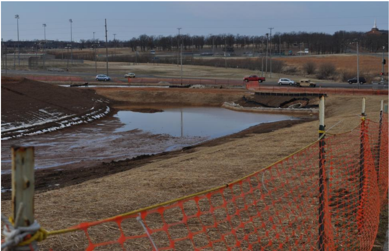
Photo 2. Current Erosion Control Problems (Corner of Nebraska and Minnesota). No silt fences, standing water, and large amounts of sediment. – Photo courtesy of USACE, Kansas City District
