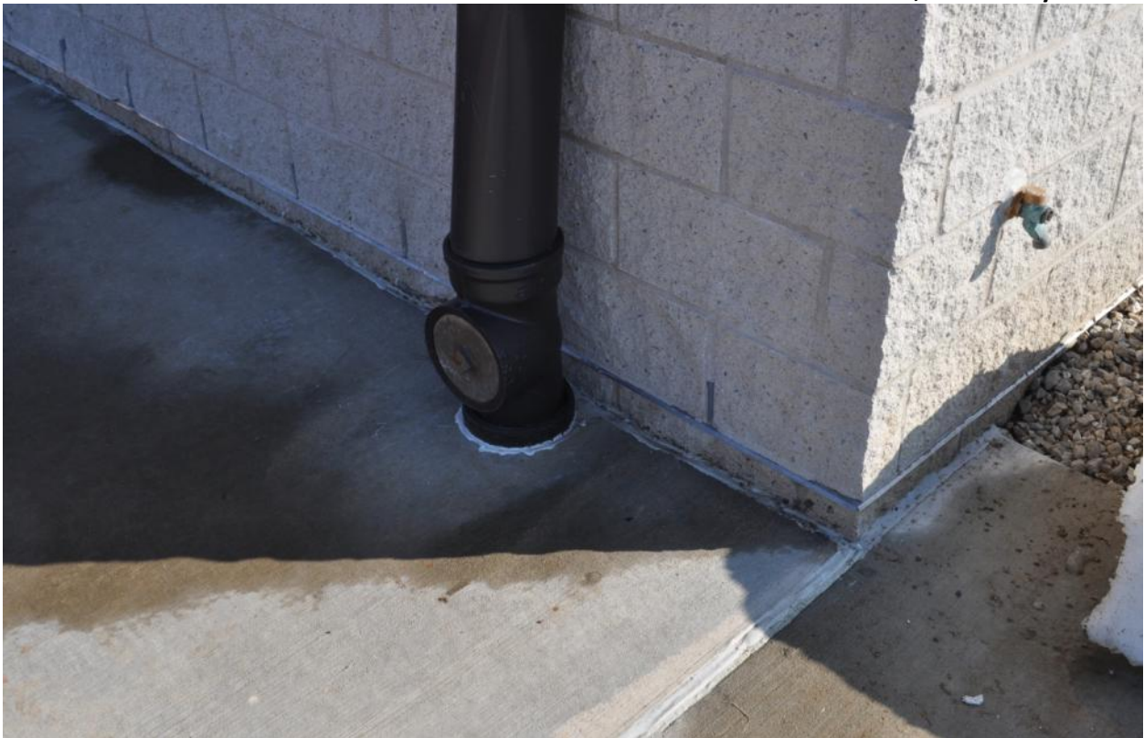
Photo 5. Example of Impervious Connections (BT Complex Roof Drain) – Photo courtesy of USACE, Kansas City District
