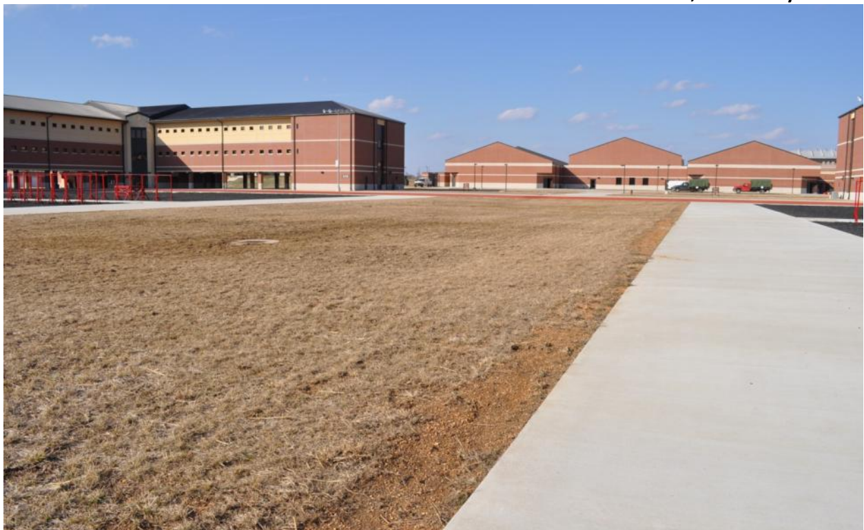
Photo 7. Poor Seeding of Grass (if any) with minimal straw covering. Construction of this complex is complete and the facility is operational, but this is all just mud with straw on top (BT Complex). – Photo courtesy of USACE, Kansas City District
