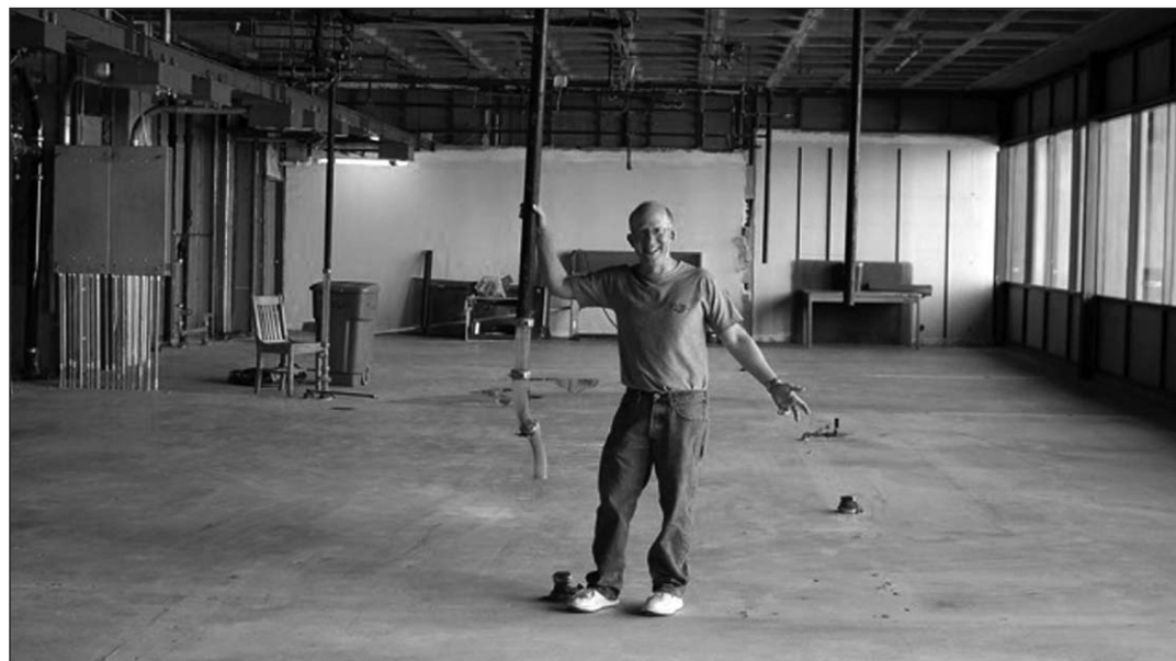
Department Head Mike Haley gestures in the site of offices and classrooms that were demolished to make way for the new general chemistry teaching labs.
