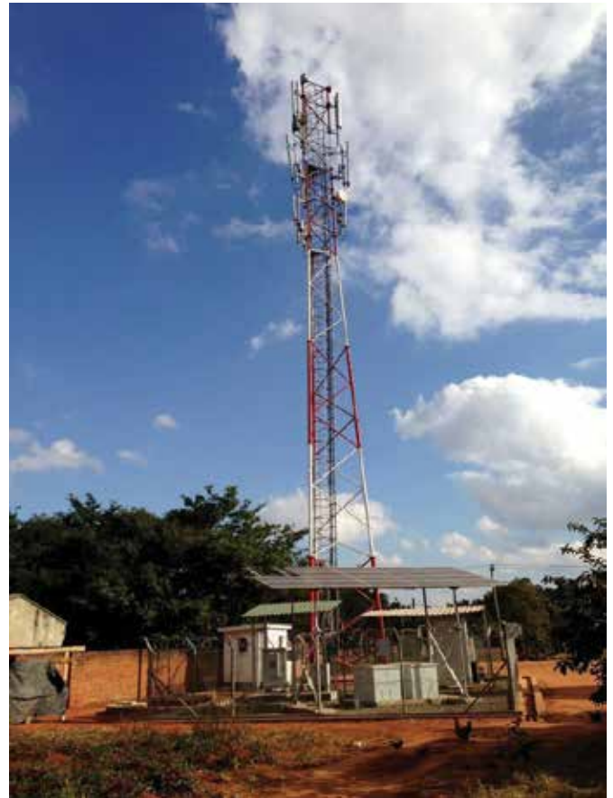
Cellular network cover is quite robust throughout Malawi, with close to 90% of the country served by two main providers. This cellular tower is in Mzuzu, forming a landmark for a neighborhood near the university campus.
