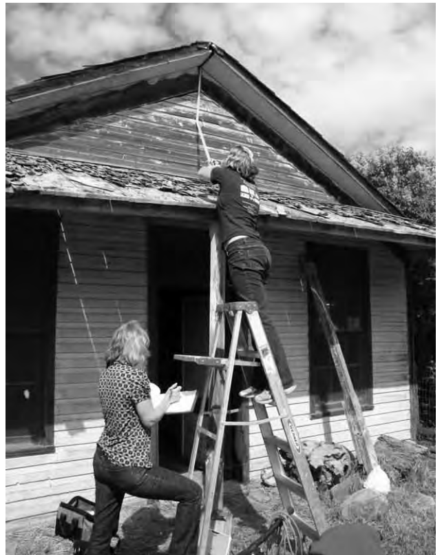
Cogswell-Taylor House (c. 1868) recordation, condition assessment, and historic context report. Graduate students Chrisanne Beckner (left) and Lisa Berenschot (right) on site, summer 2009.
