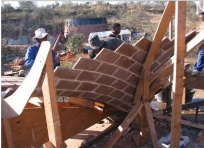
Catalan vaulting, Mapungubwe Interpretive Centre, South Africa by Michael Ramage, John Ochsendorf & others. http://www.atdforum.org/IMG/pdf_RamageATDF2010.pdf
